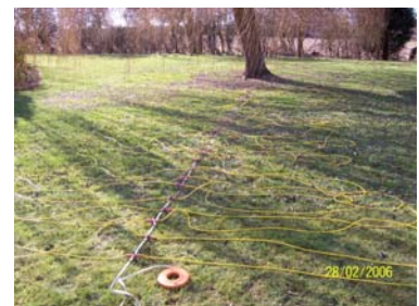
ERT Array and Cables
